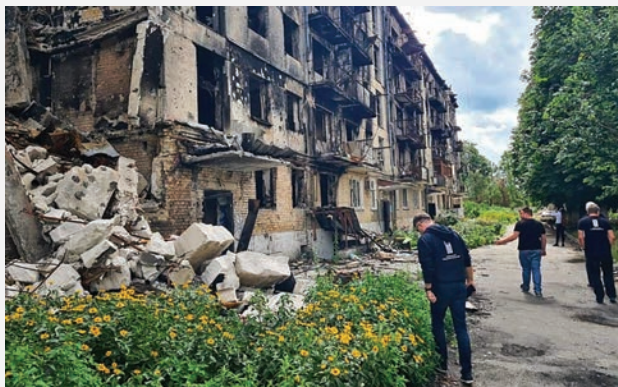
Apartment buildings have been extensively damaged by Russian rocket fire
