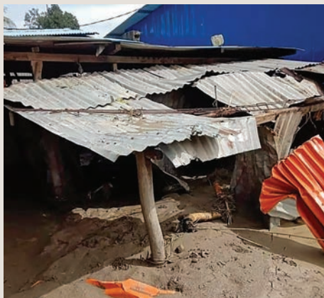
Mud damaged house
