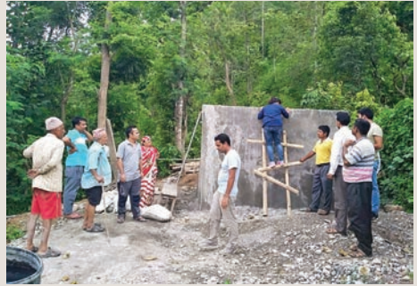
The water tank outlet in the community, connected to the solar powered irrigation pump
